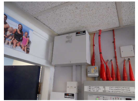
Photo 15 - Intruder alarm panel.
