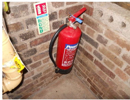
Photo 17 - Powder fire extinguisher.
