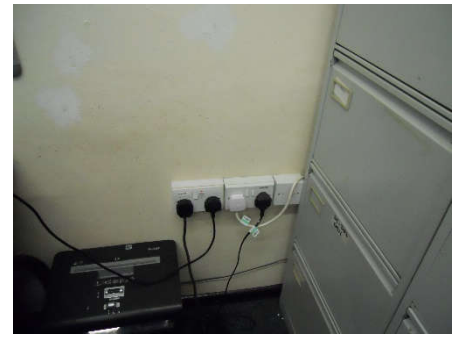
Photo 12 - Small power outlets.
