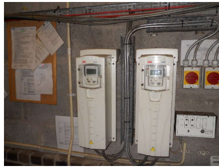
Photo 11 - ABB variable frequency inverter drives.
