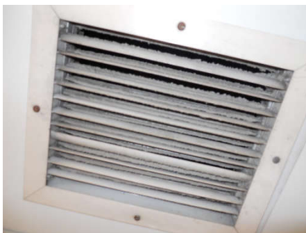
Photo 7 - Changing room extract grille and duct behind, begrimed.
