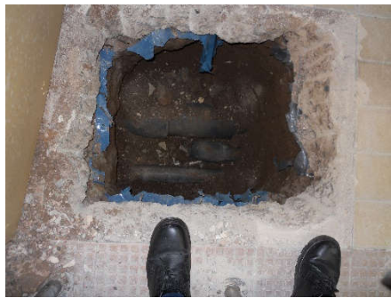
Photo 26 - Pipework to skimmers in promenade.
