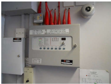
Photo 16 - Fire alarm panel.
