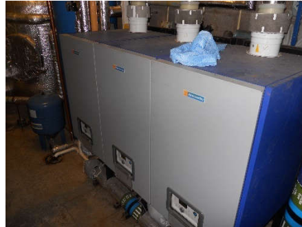
Photo 2 - LTHW heating boilers.
