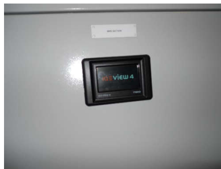
Photo 8 - Plant control panel with Trend BMS controls and IQ view 4 display.
