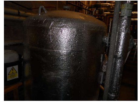
Photo 24 - Pool water horizontal multi-media filtration unit.
