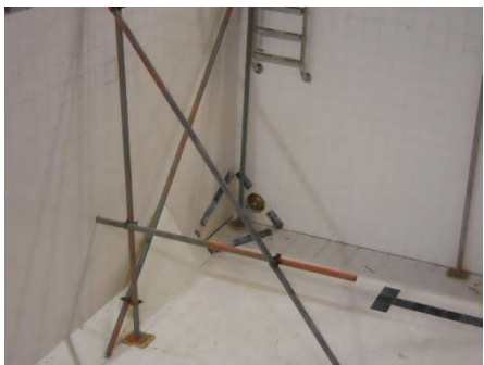
Photo 28 - Pool sump outlet, plugged.
