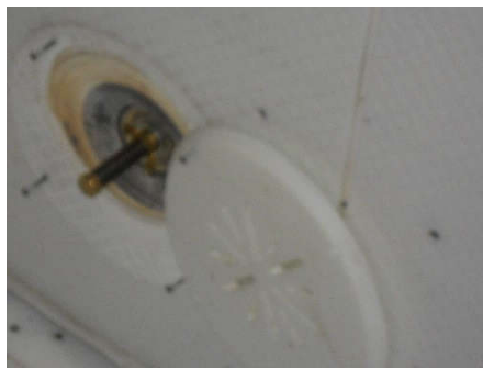
Photo 29 - Typical pool inlet with diffuser, plugged.
