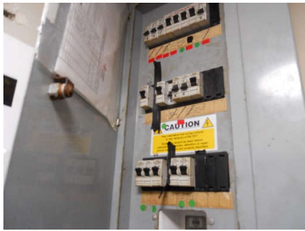
Photo 10 - Wylex distribution boards.
