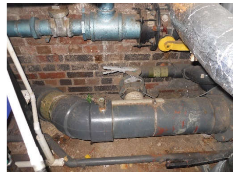
Photo 30 - Pool plastic supply pipework.
