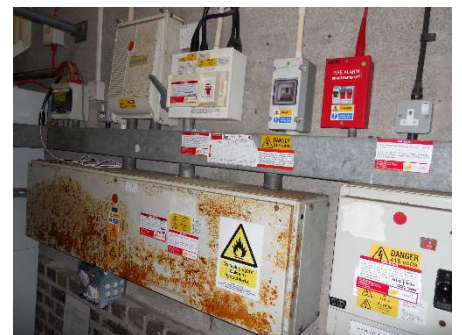
Photo 9 - Electrical bus bar with surface corrosion to enclosure.
