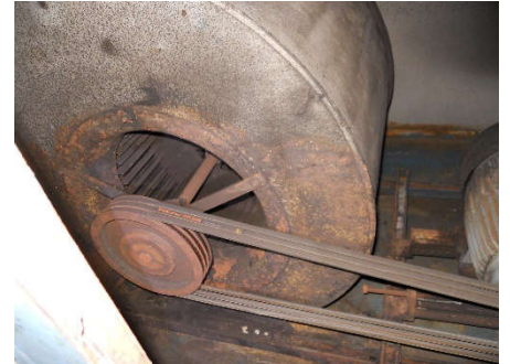
Photo 3 - Air Handling unit, extract fan with surface corrosion.
