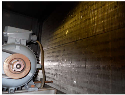
Photo 5 - Air handling unit, main heater battery with surface corrosion.
