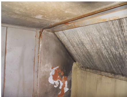
Photo 4 - Air handling unit, plate type heat exchanger with surface corrosion.
