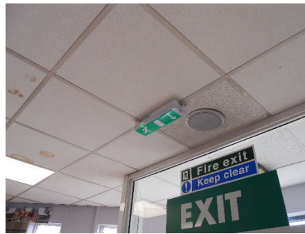
Photo 14 - Emergency bulkhead light fitting.
