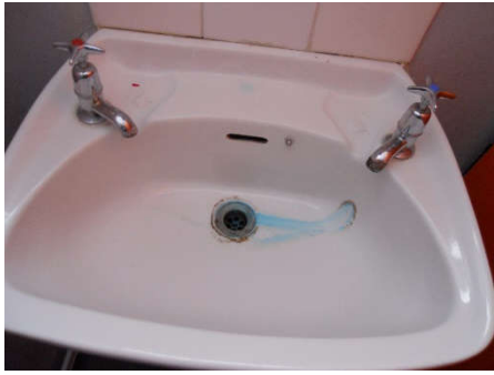
Photo 22 - Typical wash hand basin.
