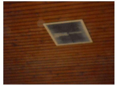
Photo 6 - Pool extract grille and ducts above, begrimed.
