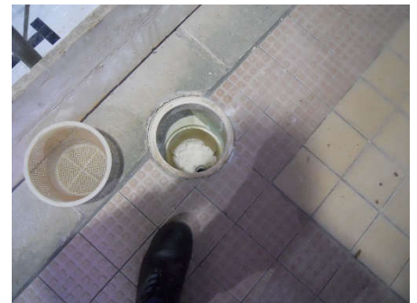
Photo 27 - Typical pool skimmer box.
